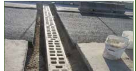
The conglomerate is removed in the vicinity of the trench where the prefabricated channel is housed.
