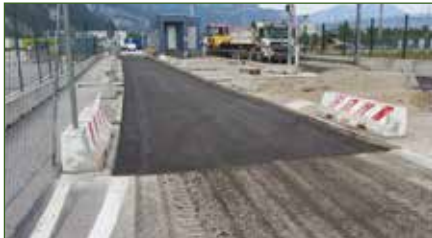
After removal of the old asphalt the strip is re-covered with a layer of cold-recycled conglomerate.
