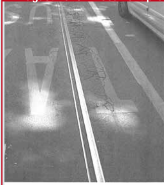
August 2015 - Recurrent problems affecting paved-in tracks
